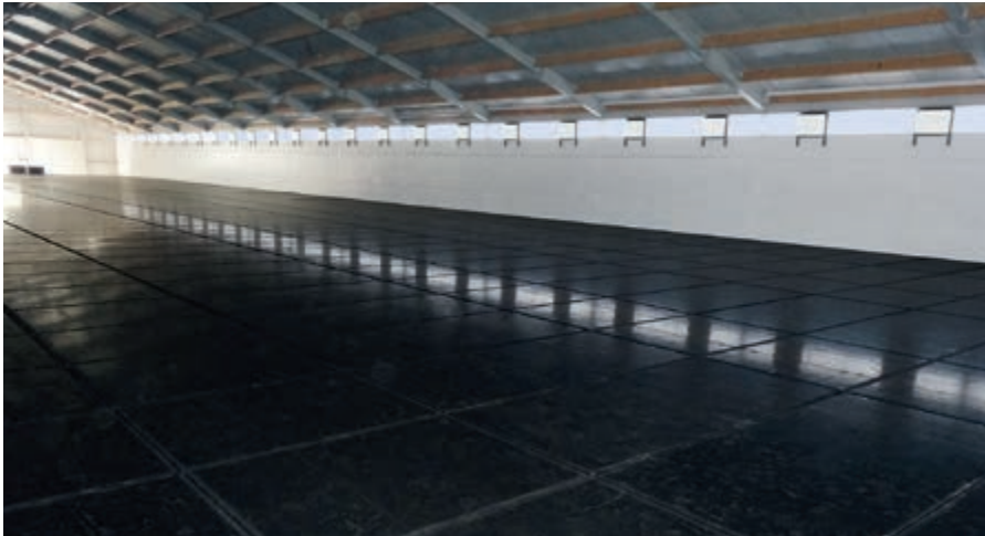
View of an intermediate ceiling made of plastic boards before the system is installed on the second level
